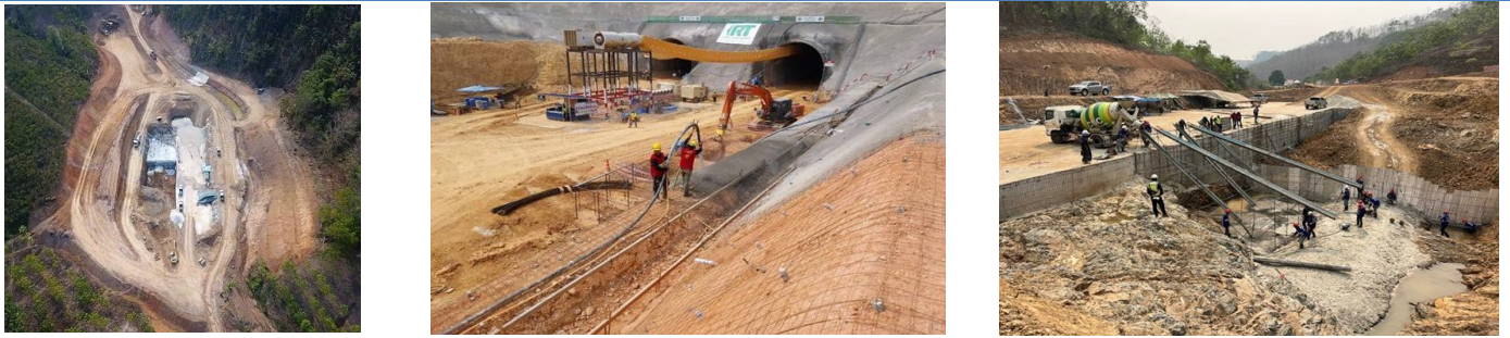
Figure 5: Ground improvement and tunnelling work for the Denchai-Chiangrai-Chiang Khong railway project (5-6% of construction progress as of Mar 2023)
